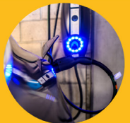
Level 2 EV Charging Stations
