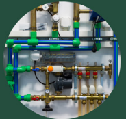
Ground Source Heat Pumps
